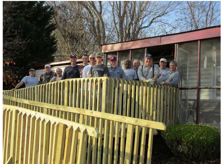
On December 1 st , the MLC Carpentry Team completed another Wheelchair Ramp for a local person in need.
