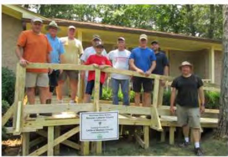
Another month, another ramp! Check out the ongoing adventures of MLC's Ramp Team at mlutheran.org/project/casa-ramp-builders/
